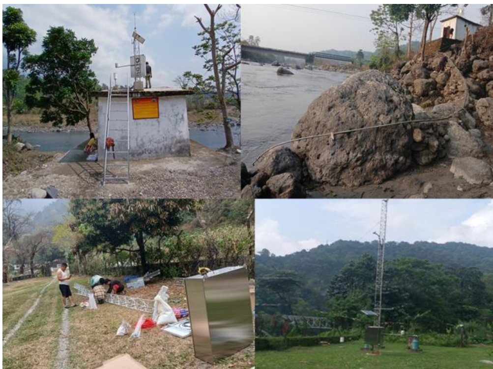
Figure 17: Photos of upgraded AWLS at Bangtar and AWS at Sershong (Gelephu)
