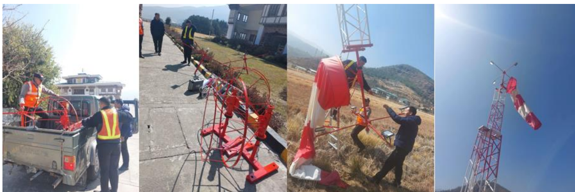
Figure 33: Flood and Obstruction lights installed at Paro and Gelephu International Airports.
