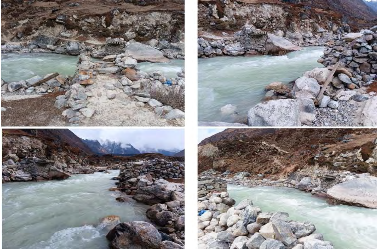
Photo 10: Damaged bridge between Tenchoe and Dota village
