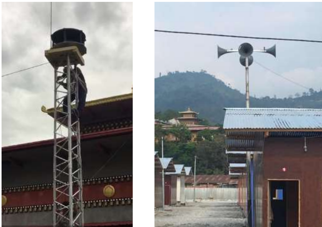
Figure 17: Warning Siren for Amochhu Settlement
